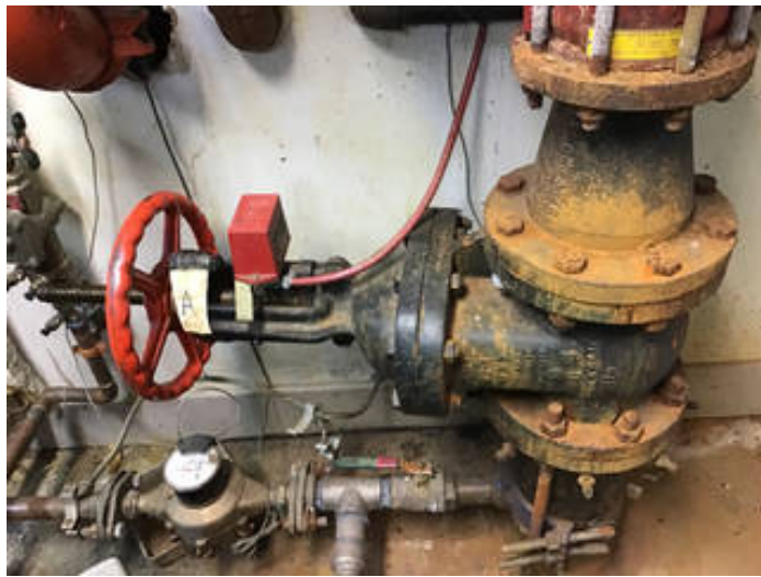
Valve - 4" Wafer Style Check Valve on Underground Sprinkler Room
