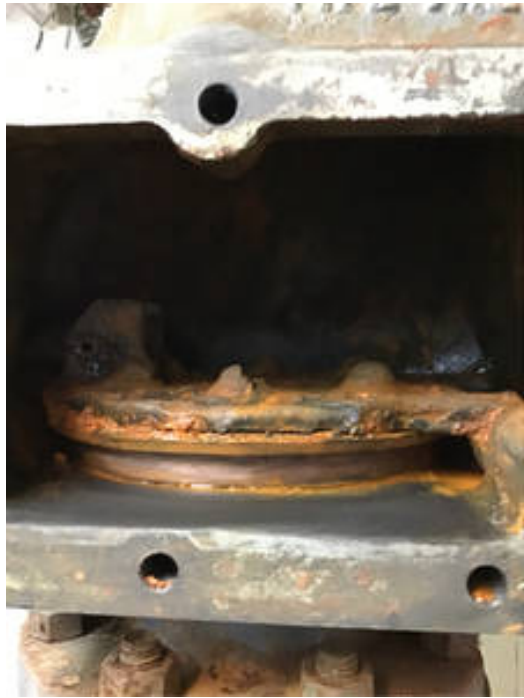
Valve - Main Control Valve Maintenance Room / Sprinkler Room
